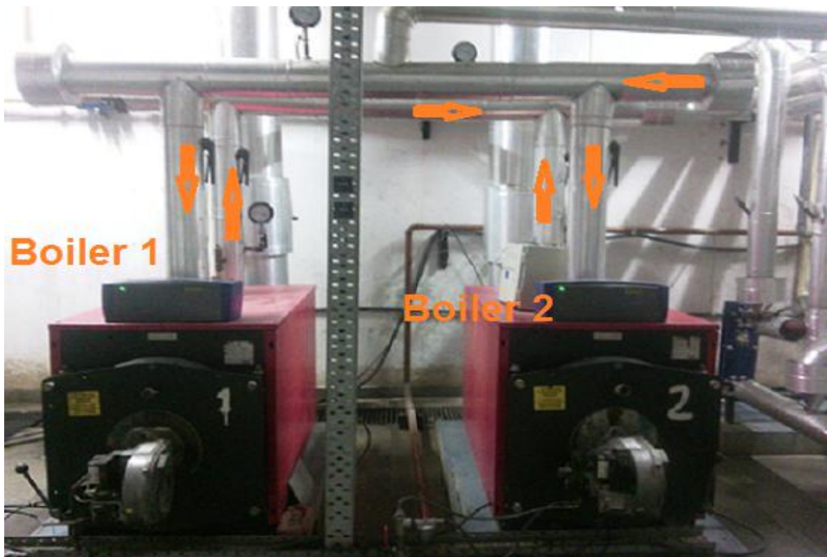
Boiler units at Hotel Roseate
