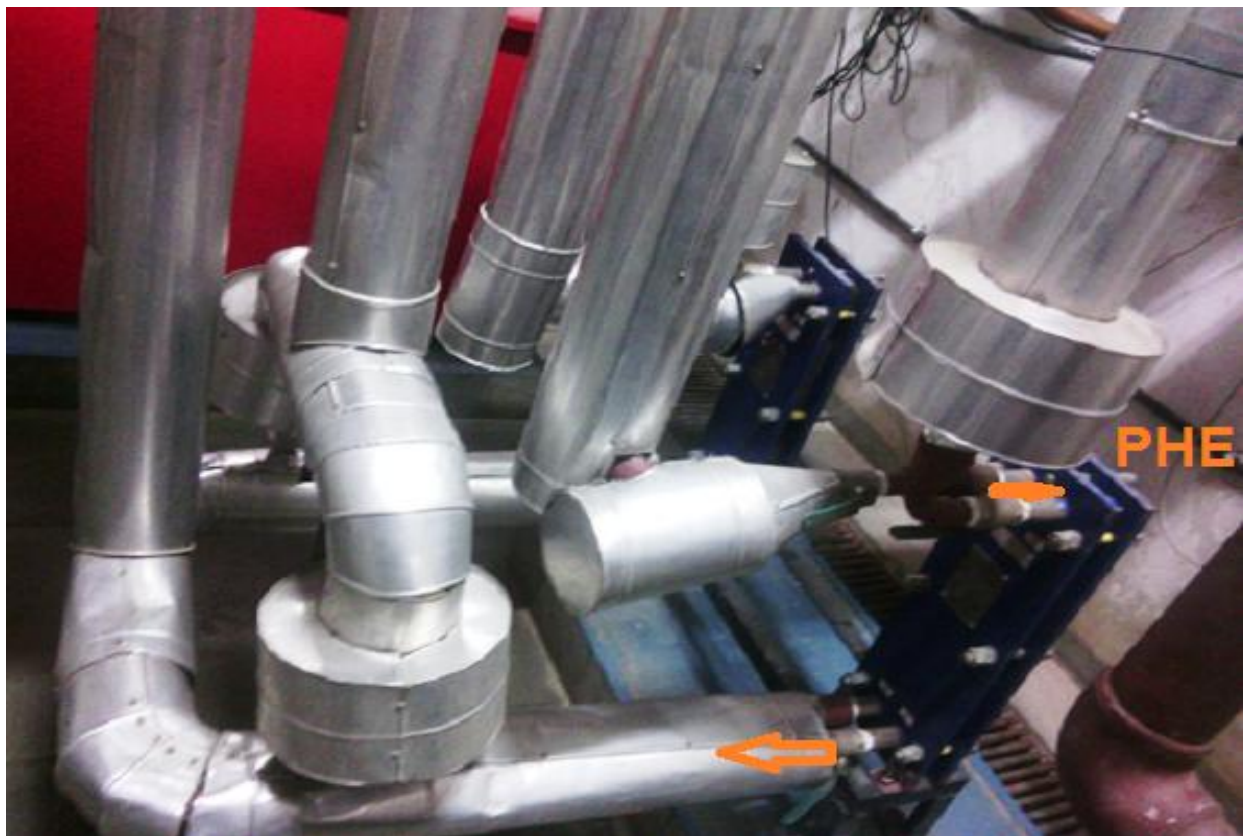
PHE system at Hotel Roseate
