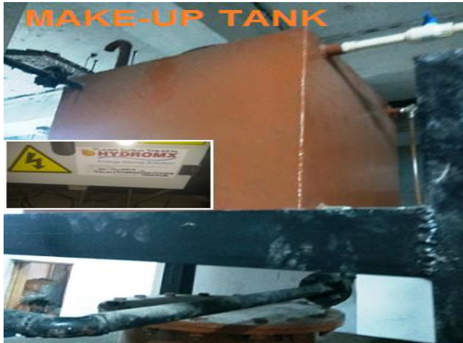
Make-up Tank at Hotel Roseate
